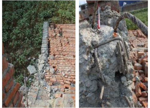
Figure 52. Cement mortar is rigid in nature and cannot withstand any major stresses/ movements lending the structure a short life span
